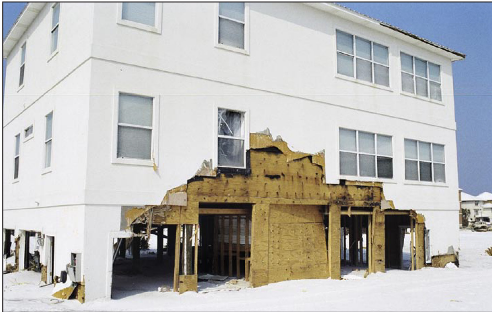
Figure 6: Damage caused by waves running up the exterior wall prior to dislodging of breakaway walls during Hurricane Ivan in 2004 (Pensacola Beach, FL)
