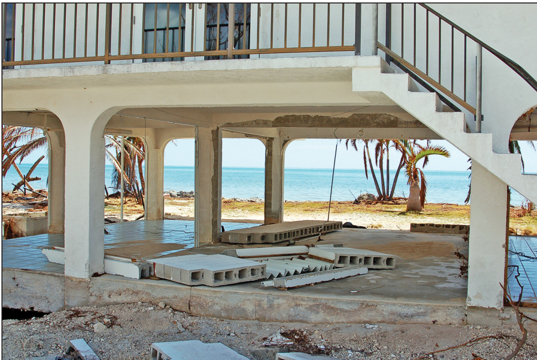
Figure 5: Unreinforced masonry breakaway walls removed by waves (i.e., performed as intended) during Hurricane Irma in 2017 (Monroe County, FL)
