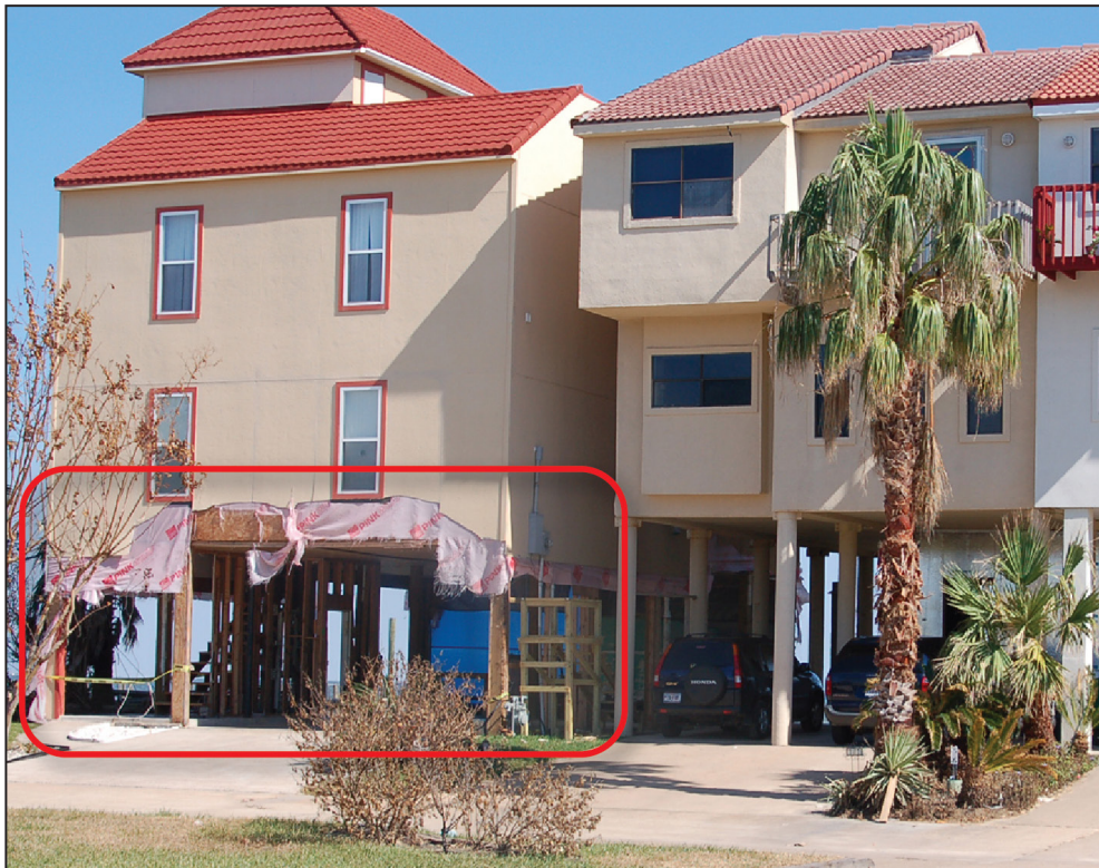
Figure 7: Non-compliant joint detailing, resulting in the propagation of damage above the lowest floor when the breakaway walls broke away during Hurricane Ike in 2008 (Seabrook, TX)
