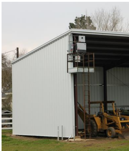
Figure 24: Elevated Electric Service and Equipment
